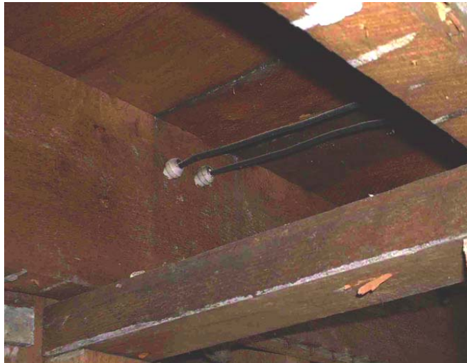
Fig. 1a – Knob-and-Tube Wiring From House IL-6
