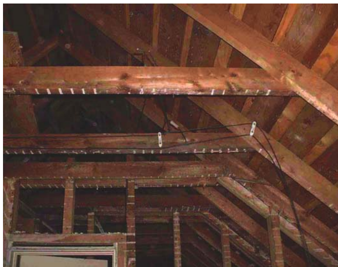
Fig. 1b – Knob-and-Tube Wiring From House IL-6
